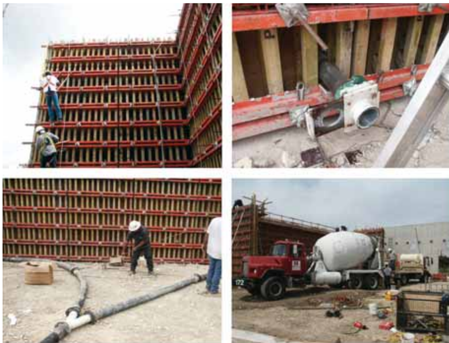
Figures 3–6 clockwise from top left: Erecting second side of wall formwork; Port for pumping concrete from bottom; Pumping concrete into wall formwork from bottom; Splitting concrete flow to two ports.
